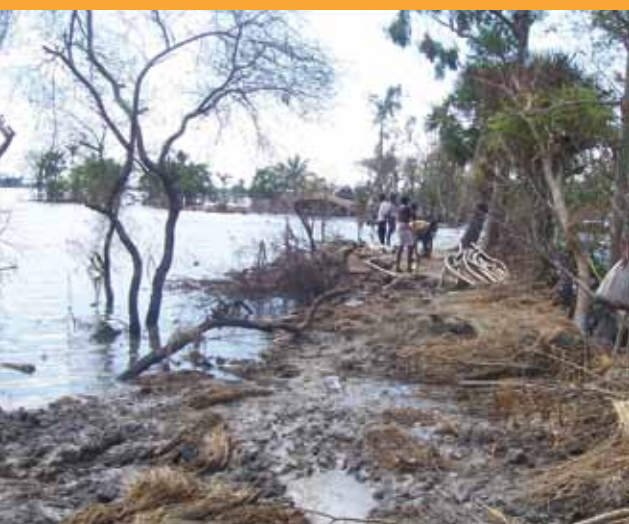
Embankment Damage in Indian Sundarbans after Cyclone Aila.
